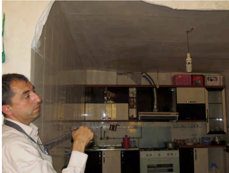
Figure-10: Damage to the buildings in Abanar: collapse of walls, figures and object and plaster fall in the kitchen.
