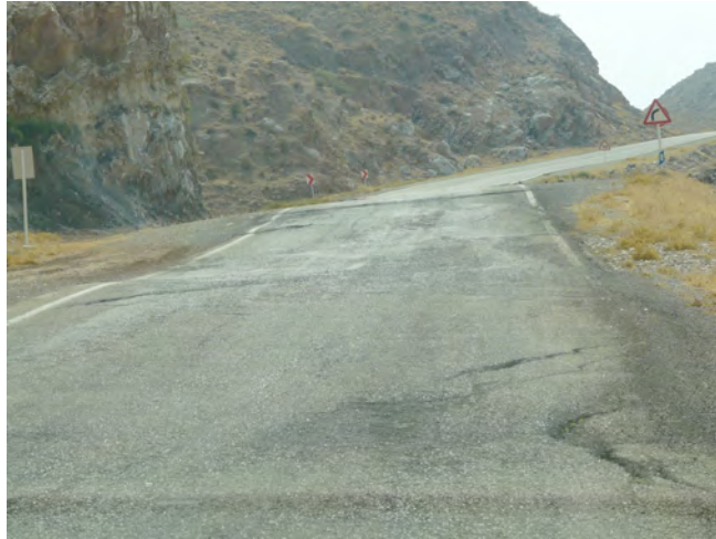
Figure-8: Road from Darreh-Shahr to Abdanan (32km from Darreh-Shahr): Fissures and land subsidence caused by the 18 August 2014 earthquake (about 42km distance to epicenter).
