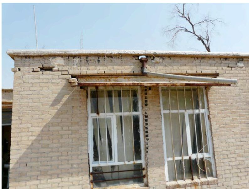
Figure-9: Damage to a building in Mormori.
