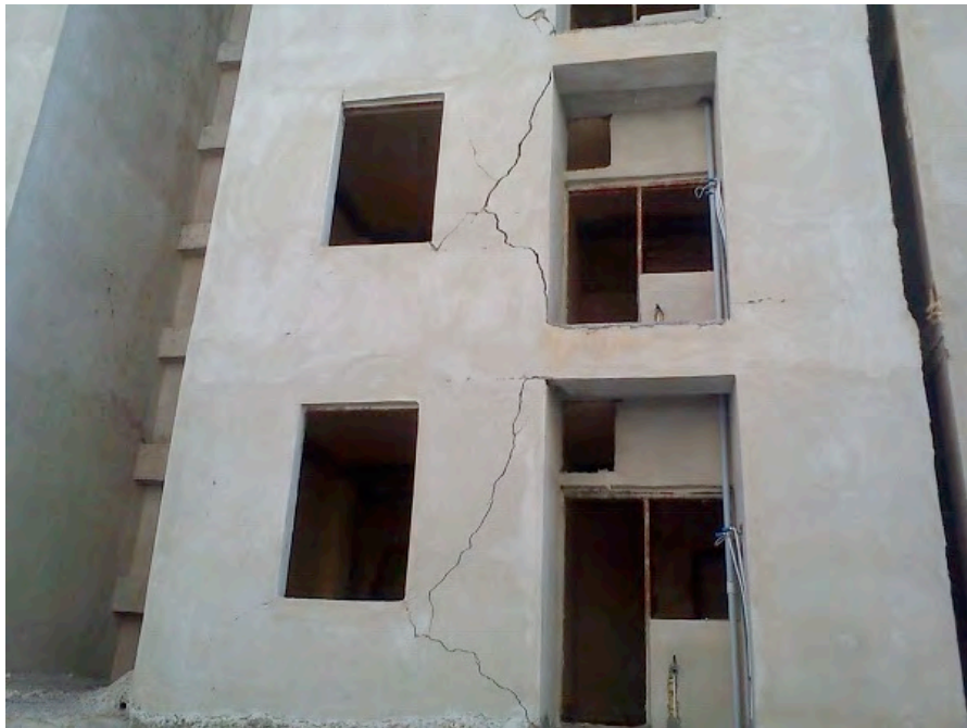
Figure-11: Cracks created in "Mehr" Apartments (Maskan-e Mehr) in Abdanan (38km from the epicenter); constructed about one year ago and suffering extensive damages due to an intensity VI (EMS98) in the 18 Aug 2014 Mormori earthquake.
