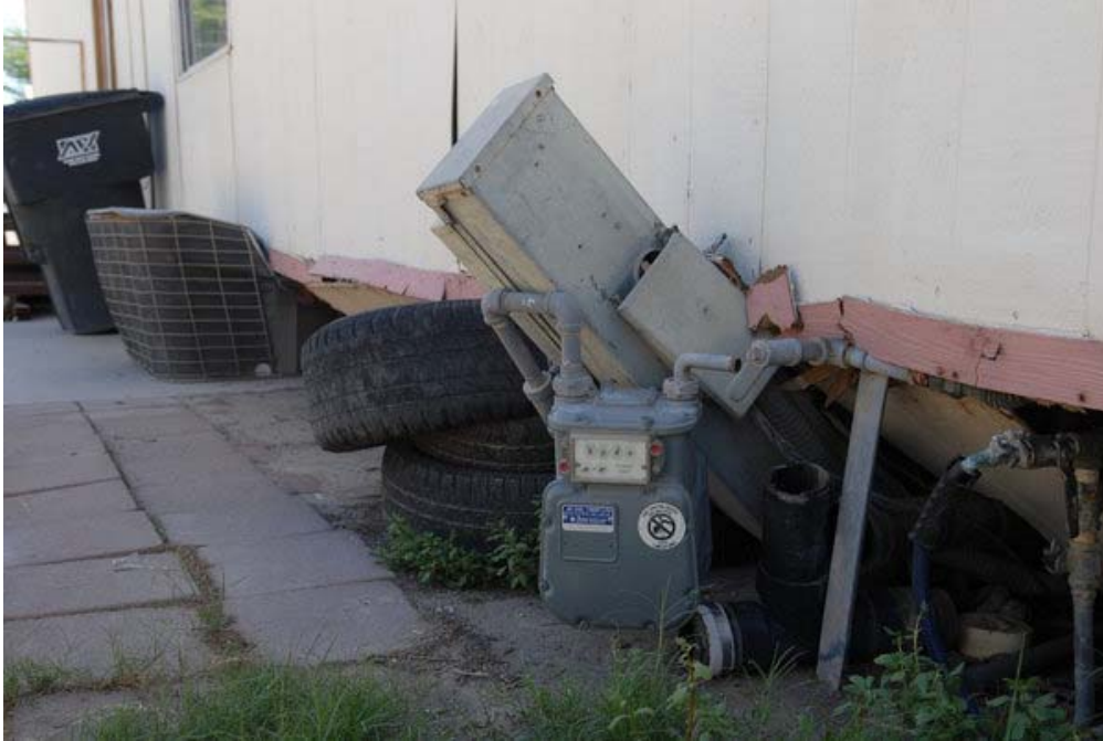
Mobile home in Brawley displaced off its blocks. Air conditioner in background, gas meter, etc. were damaged.
