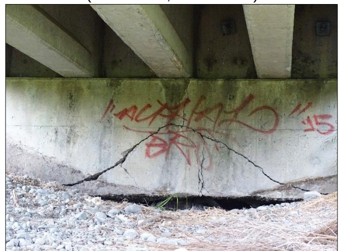
Damage to the Waiau River bridge #1842 abutment (evidence of ground movement in the vicinity) (-42.655495, 173.031173)
