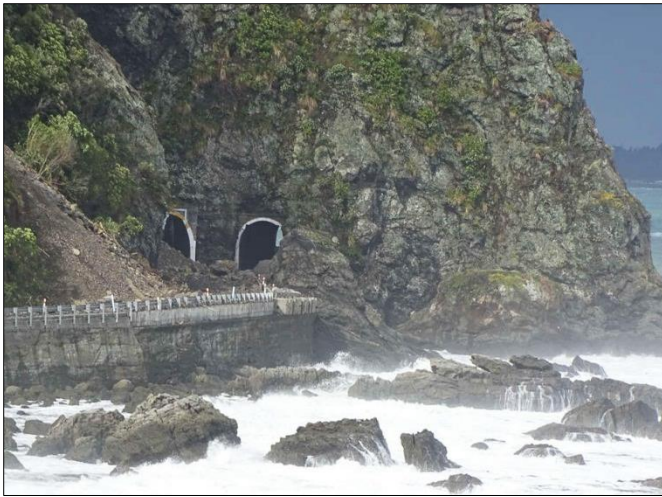
(d) Blockage of tunnel entry due to rock fall, looking south
