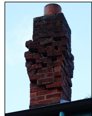
Extensive dislodgment of the bricks, Hanmer Springs
