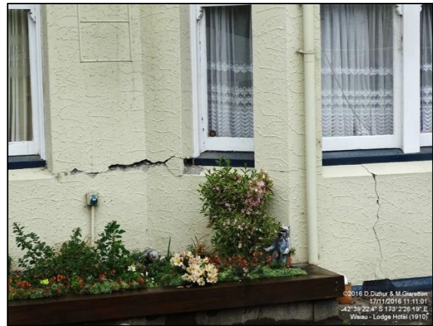
Horizontal cracking showing evidence of pier rocking
