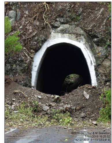
(e) Entry tunnel blocked due to rock fall, looking south
