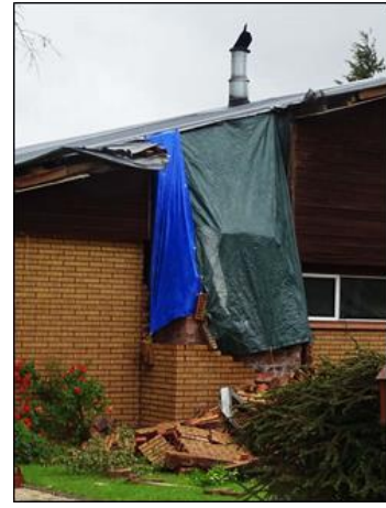
Collapse of moder brick veneer and chimney, Waiau
