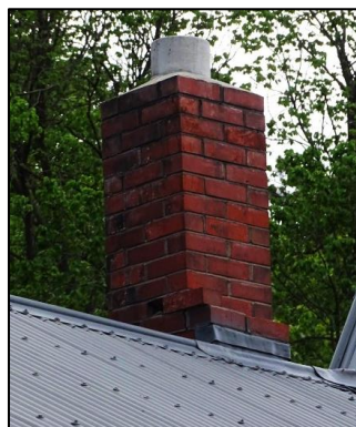
Horizontal crack at the chimney base and sliding, Hanmer Springs
