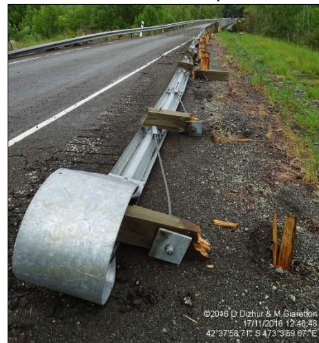
Breaking of the railing supports due to significant displacements of the deck structure
