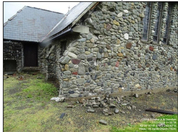
Significant cracking of corners and gable wall
