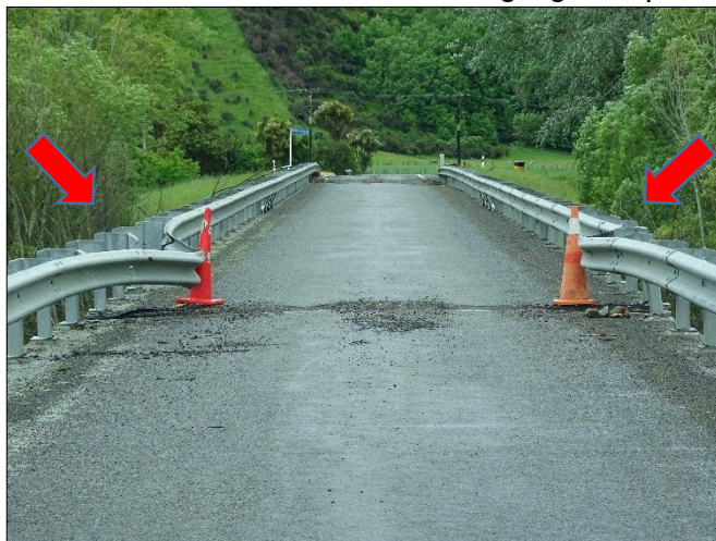
Buckling of the bridge side railing due to deck movements
