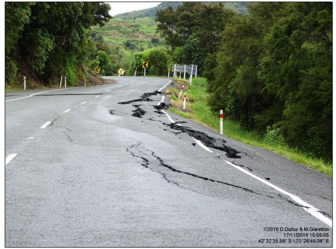
Significant road pavement deformation near SH1
