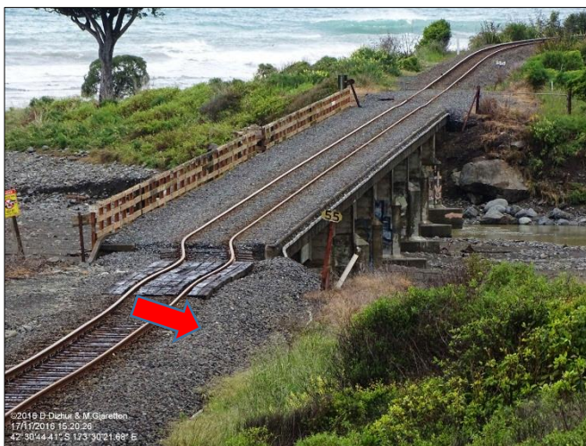
Lateral movement of the bridge abutment, not observed damage of the bridge structure (-42.513496, 173.506657)
