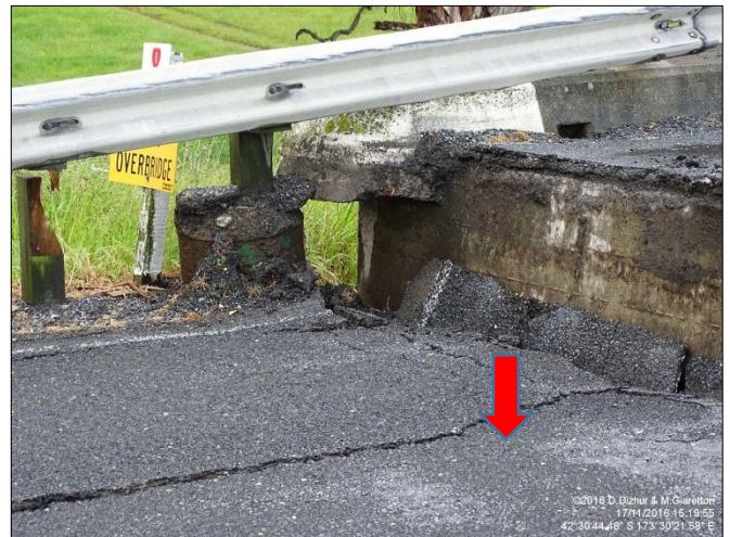
Upto 1.0 meter of differential movement observed
