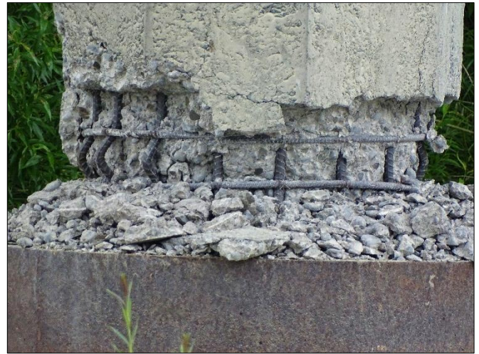
Significant spalling at the base of column (southern column). Longitudinal reinforcing bar buckling
