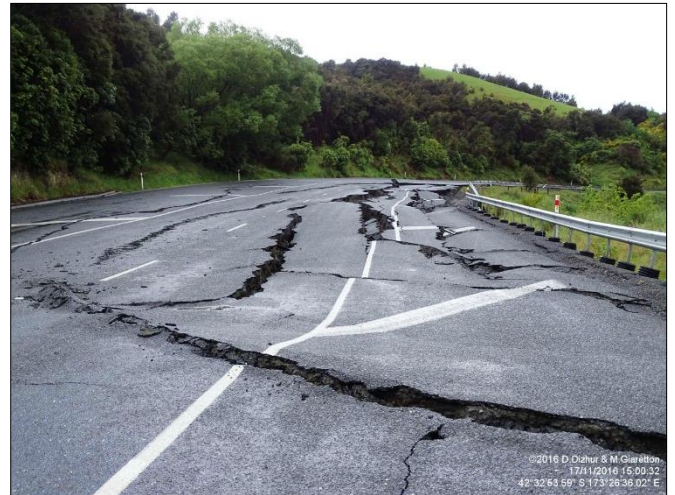
Significant damage to the road pavement
