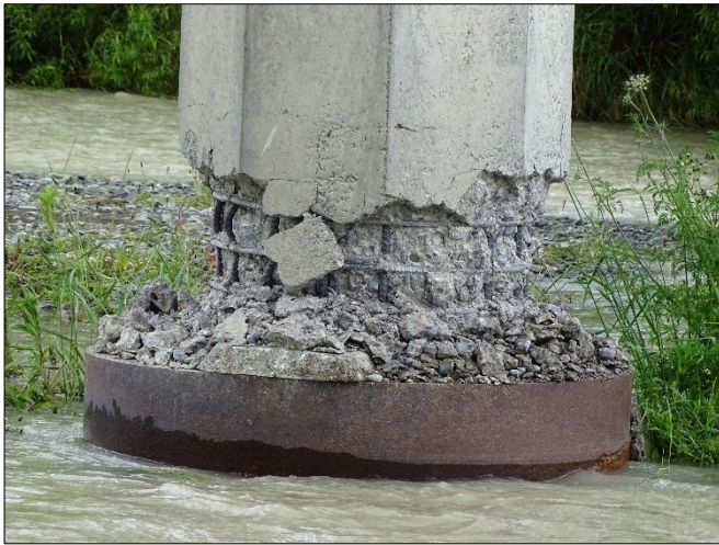
Significant spalling at the base of column. Longitudinal reinforcing bar buckling
