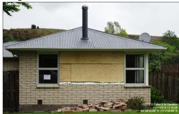
Collapse of large veneer panels, Waiau
