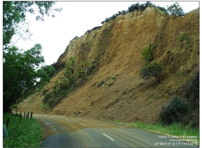
Major rock fall on Leads Road
