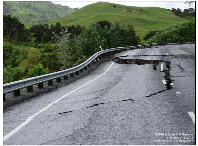
Movement of pavement due to land sliding below
