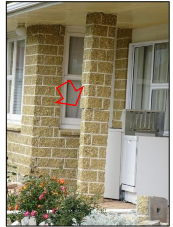
Torsion of the top part of the column, Seddon
