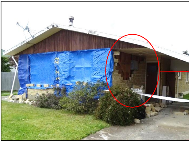
Out-of-plane collapse, Seddon
