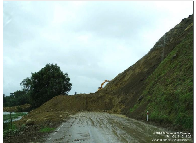
Land slide being cleared SH70 towards Waiau (by pass available)
