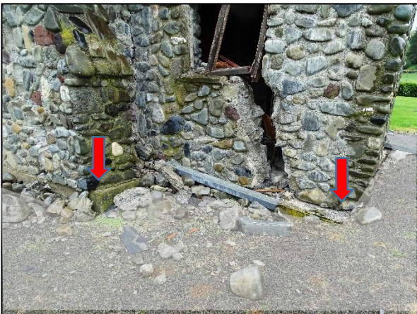
Close-up of the significant bearing failure of tower foundation
