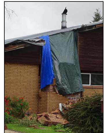
Collapse of the chimney stack, Waiau
