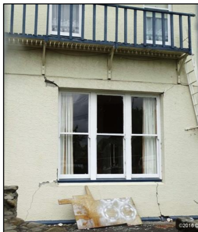
Cracking around widow openings
