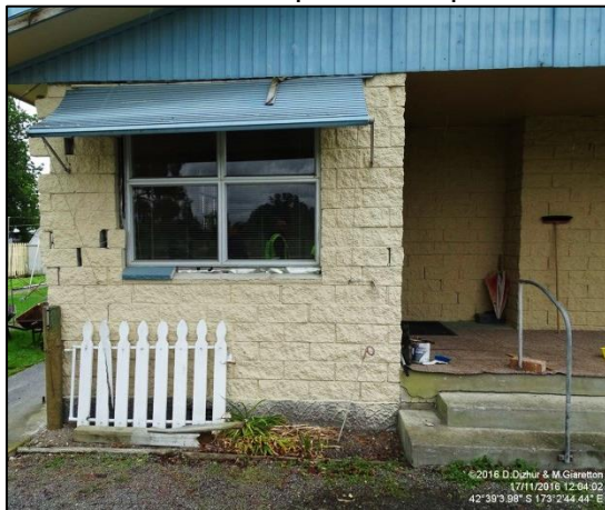
Significant damage to veneer dwellings, Waiau
