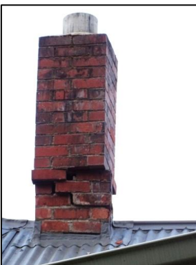
Horizontal crack at the chimney base and torsion, Hanmer Springs
