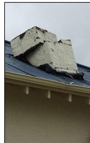
Partial collapse of chimney
