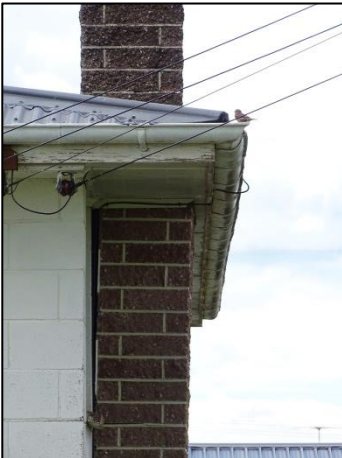
Out-of-plane detachment of the chimney stack, Seddon
