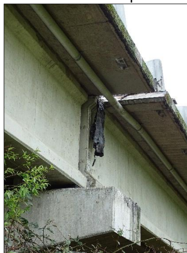
Significant differential movement of bridge girders
