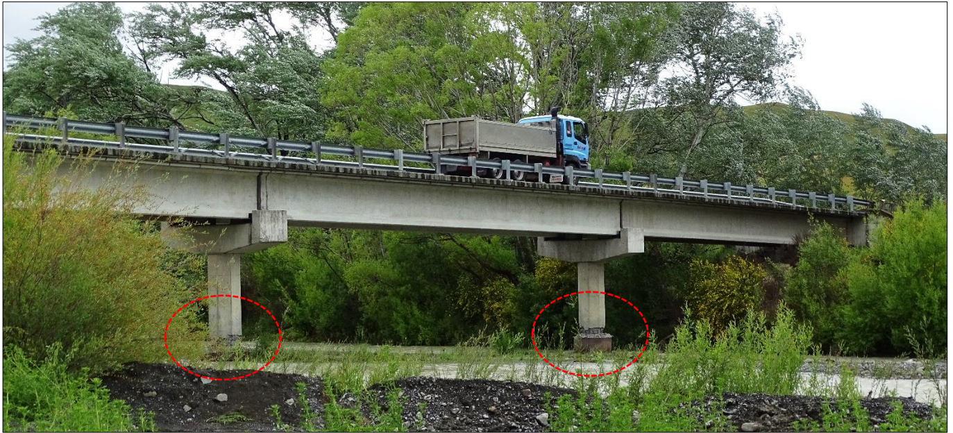
Bridge along Inland Road, open for emergency heavy vehicles. Major damage to the bridge structure, all columns showing signs of plastic hinges (-42.634382, 173.066299)
