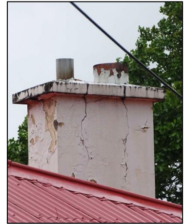
Vertical crack-pattern, Waiau
