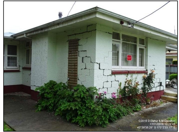
Concrete blocks building, extensive cracking and dislodgment of the blocks, Waiau
