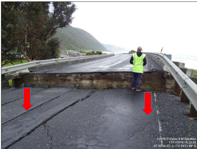
Major settlement of abutments, Oaro overbridge #1790 (-42.512124, 173.506385)
