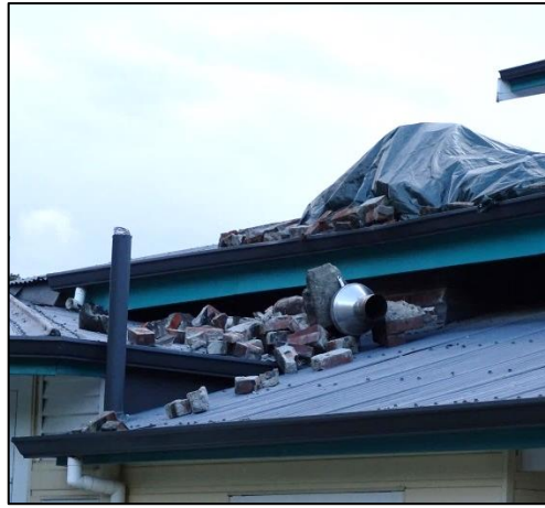
Collapse, Hanmer Springs
