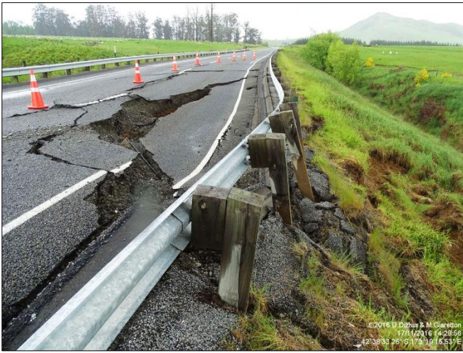
Landslide into a creek below. State Highway 1, north of Leads Road
