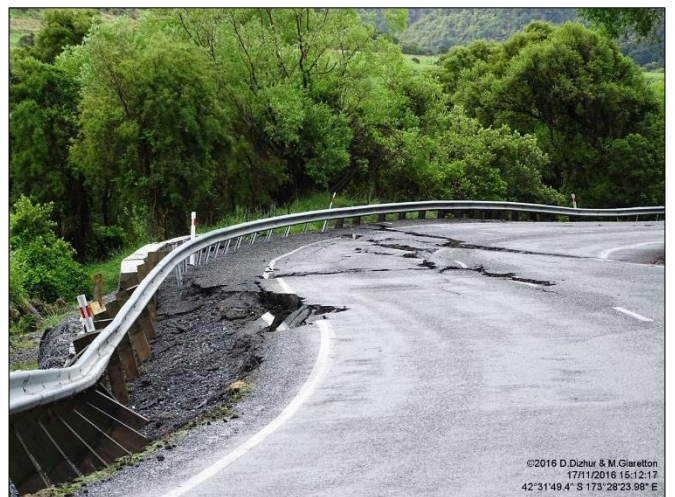
Significant damage to the road pavement and railing
