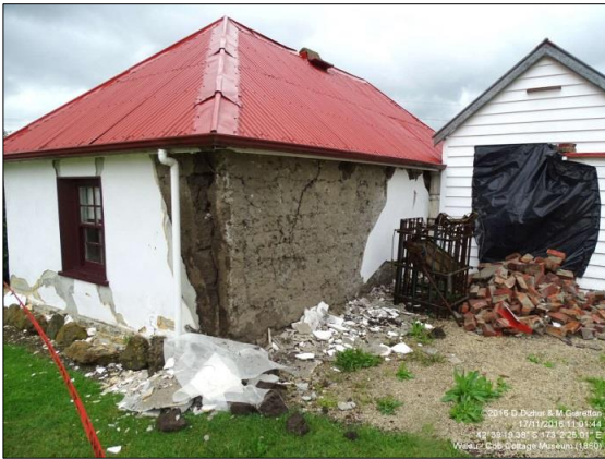
Damage to the Cob Cottage museum
