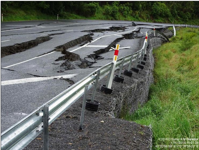
Significant damage to the road pavement and movement of retaining structure
