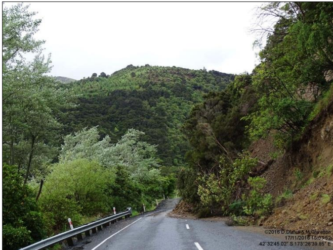
Major slide along SH1
