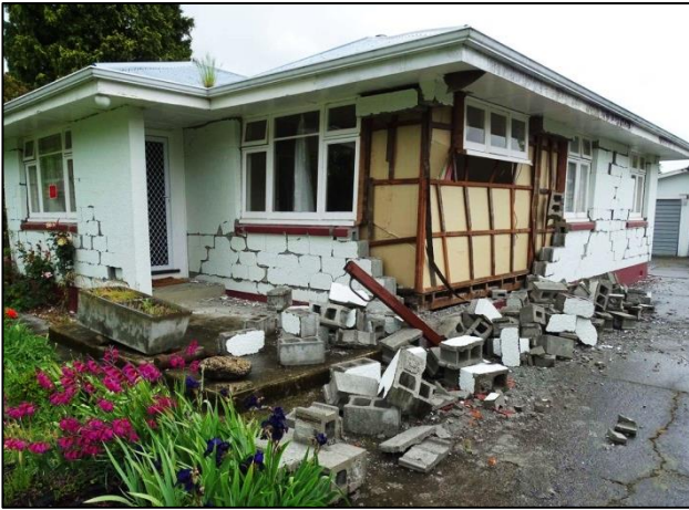
Concrete blocks building, out-of-plane collapse, Waiau
