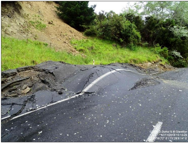
Major bulging of the road pavement due to land slip above
