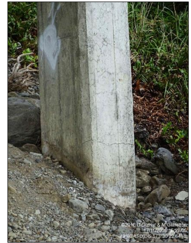
Signs of hinging at the column base
