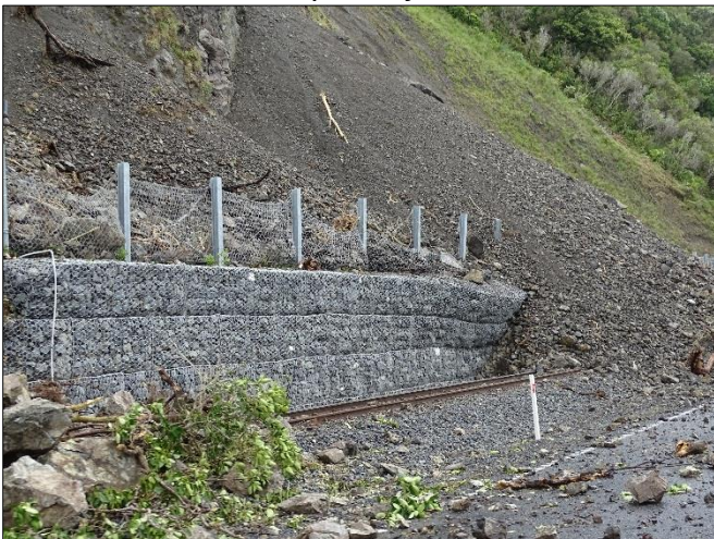
(c) Damage to retaining structure and rock fall protection system
