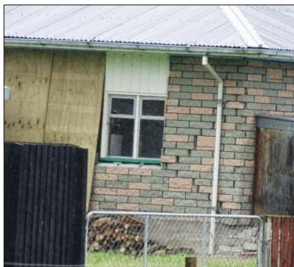
Corner damage and collapse of large veneer panels, Waiau
