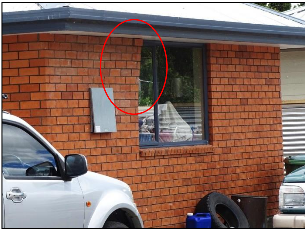
Detachment at the top of the veneer wall and initiation of out-of-plane collapse, Seddon
