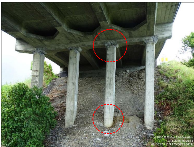
Under bridge deck, visible hinging of the columns
