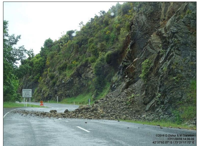
Example of typical rock fall on SH1, numerous cases along the stretch of road from Chevron to Kaikoura
