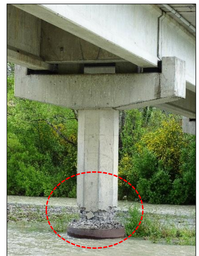
Hinging of bridge columns (see close-up)
