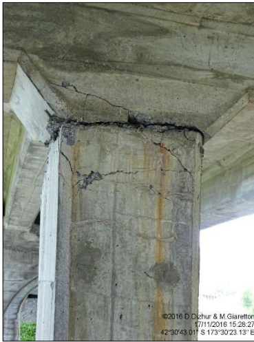
Plastic hinging at the top of column
