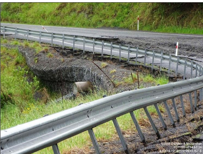
Major movement of a retaining wall
