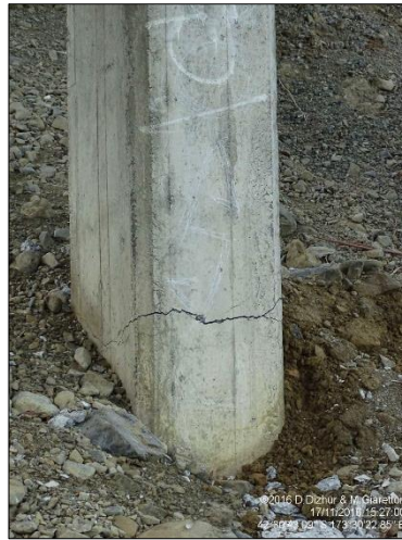
Signs of hinging at the column base
