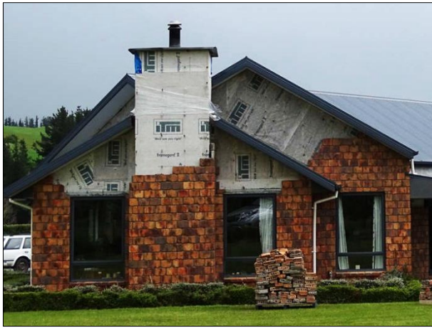
Collapse of moder brick veneer system, Waiau
