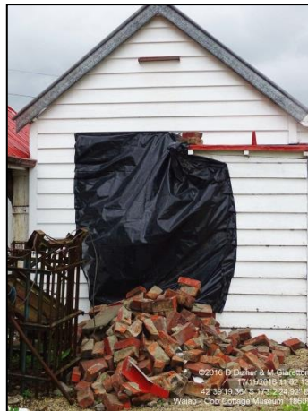
Full collapse, Waiau
