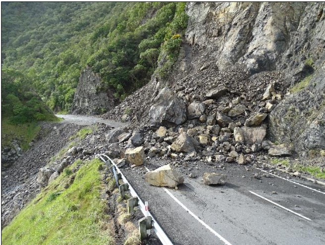
(b) Major rock fall over SH1 – attempts were been made to partially cleared
