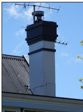
Horizontal crack at the base, Blenheim
