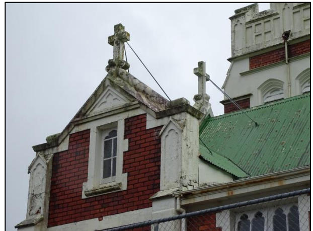
Presence of existing damage (cracks and deteriorated bricks)
