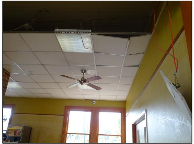
Ceiling damage due to chimney
