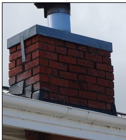
Dislodgement of the bricks, Blenheim
