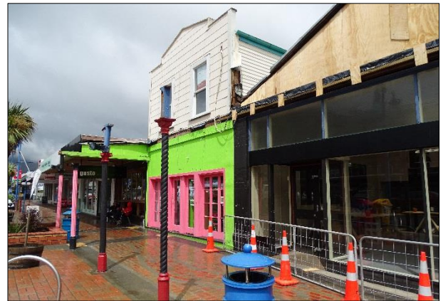
Collapse of front façade and canopy – all cleared and removed
