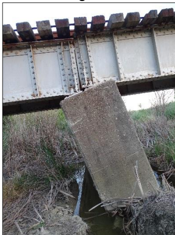
Major railway bridge pier rotation
