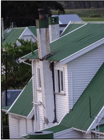
Out-of-plane detachment of the chimney stack, Clarence
