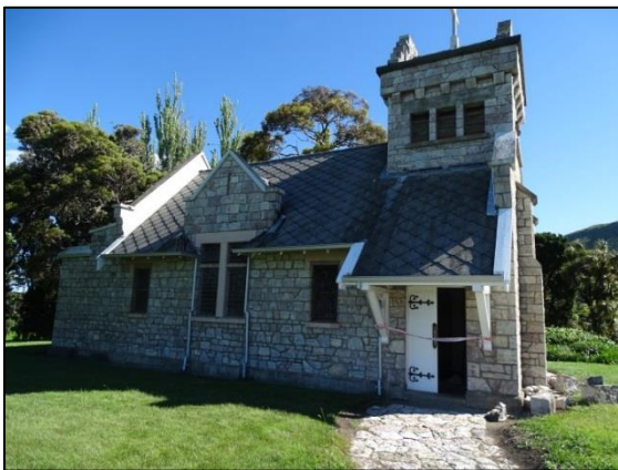
St Oswald's Church, stone and concrete, collapse of parts of front parapet
