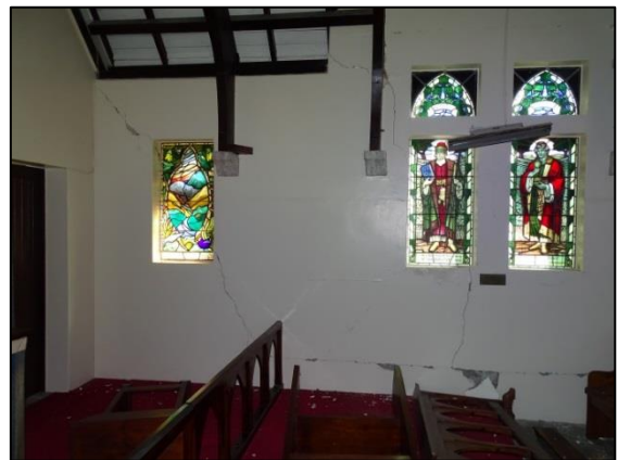
Internal view with diagonal shear and shear sliding cracks
