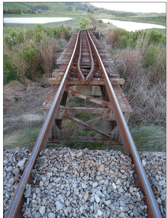
Major horizontal and vertical movement of land near bridge
