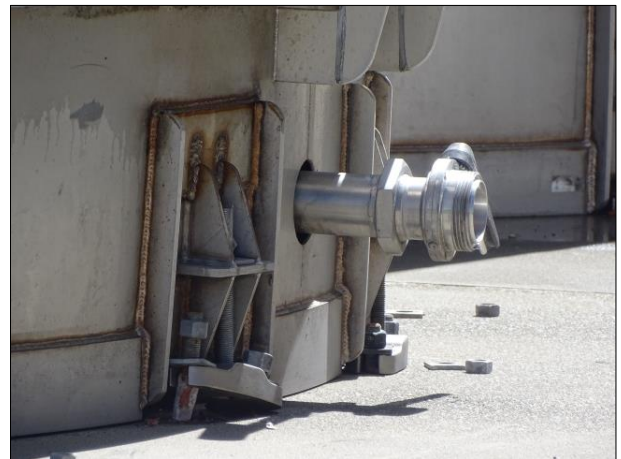
Pull-out of some adhesive anchoring connection
