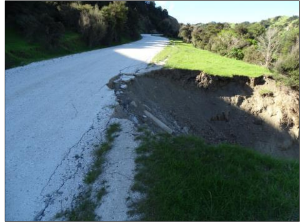
Typical condition of nearby rural roads - 100s land slips
