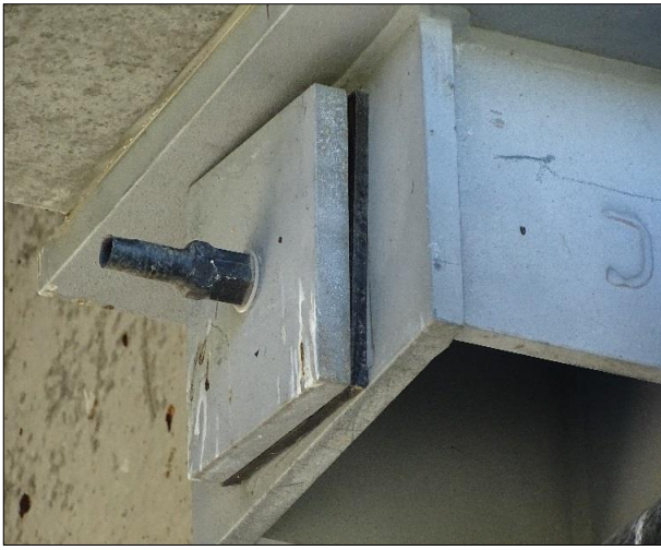
Evidence of plate movement and losing of connections
