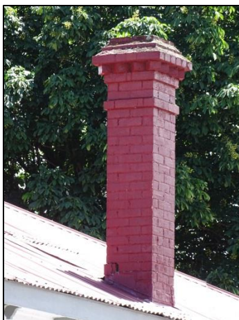
Horizontal crack at the chimney base and torsion, Blenheim
