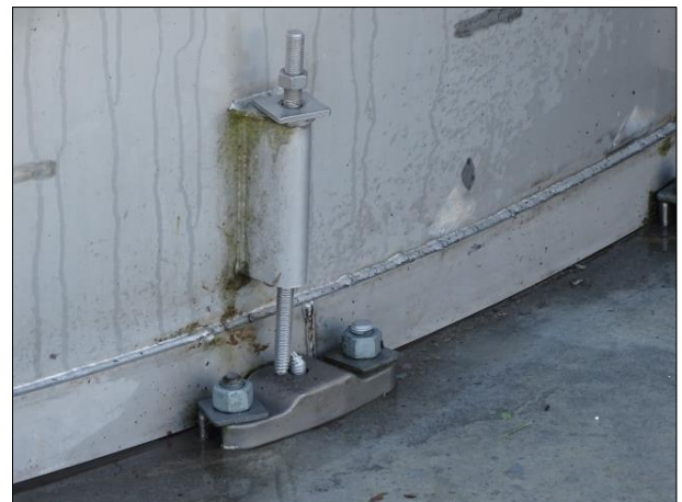
Shear failure of connection rods
