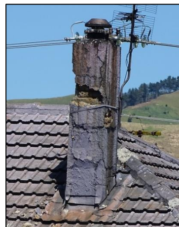
Extensive damage of the plaster, Blenheim
