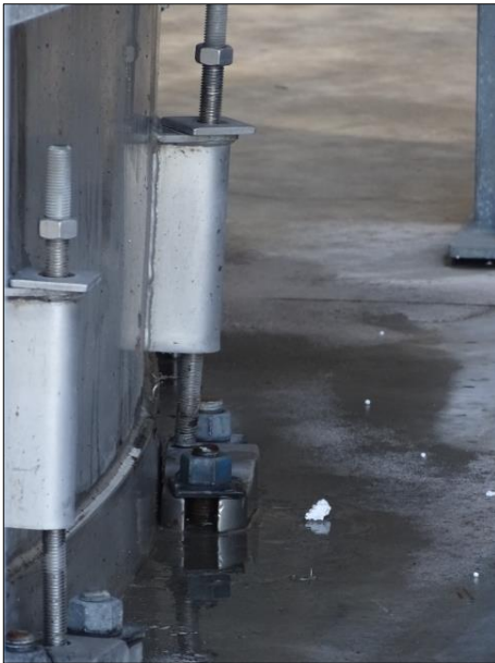
Shear failure of connection rods
