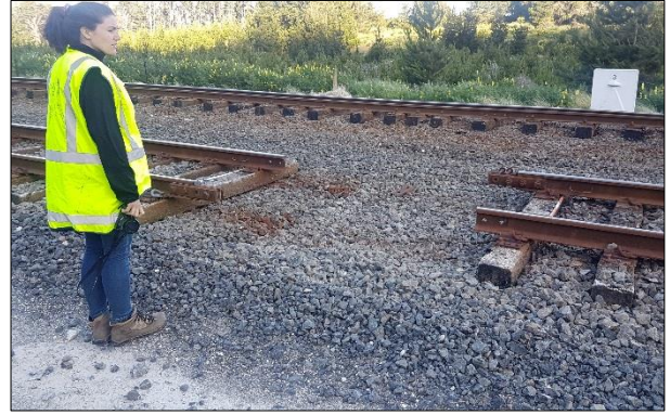
Shear failure and spread of railway lines
