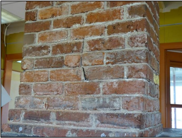
Chimney internal stack, torsional damage
