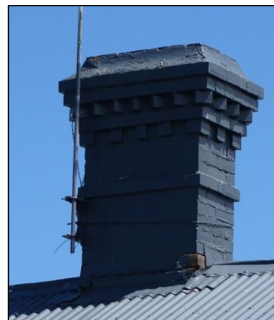
Horizontal crack at the roofline, Blenheim
