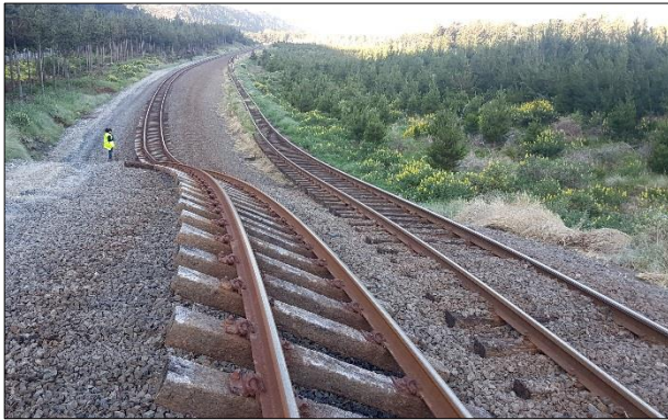
Major lateral displacement of railway lines
