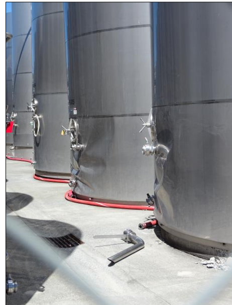
Tank buckling observed
