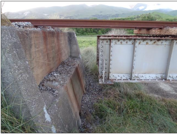
Bridge movement over one meter away from abutment
