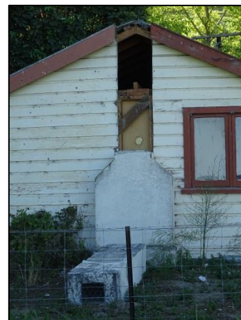
Outward collapse of the chimney stack, Clarence
