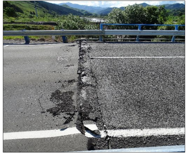
Damage to south approach
