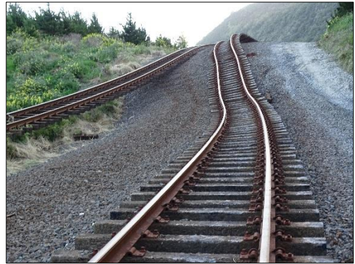
Major lateral displacement of railway lines
