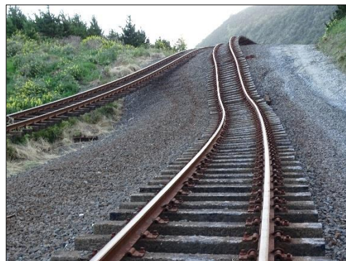
Major lateral displacement of railway lines
