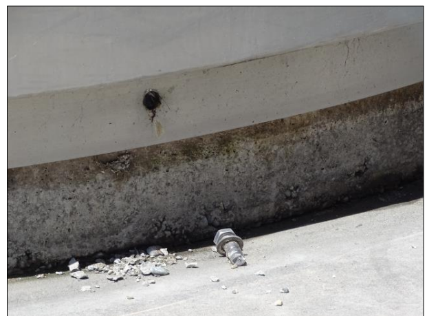
Shear failure of tank connections
