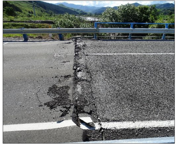
Damage to south approach
