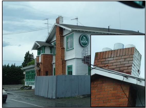
Junction Hotel – movement of chimney
