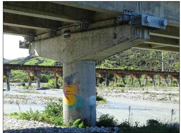
Evidence of pier inclination towards west
