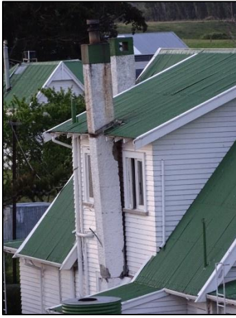
Out-of-plane detachment of the chimney stack, Clarence
