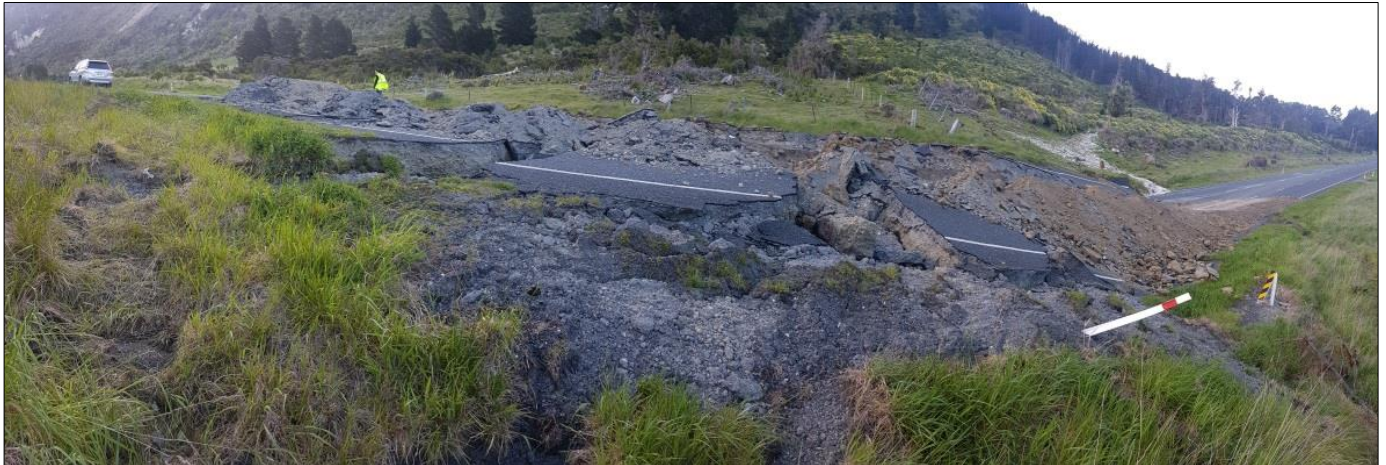
Meteres of vertical uplift, road completely destroyed – 4WD access across
