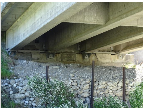
Minor concrete spalling at south abutment
