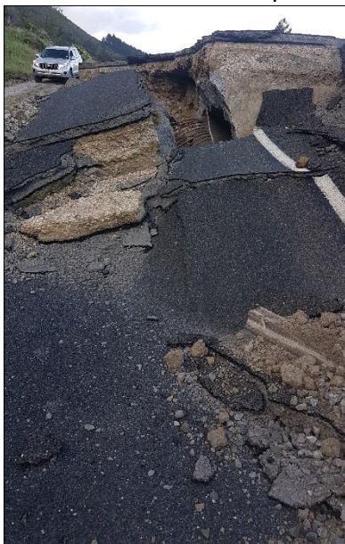
Upto 3 meters of vertical drop in road level (looking north)
