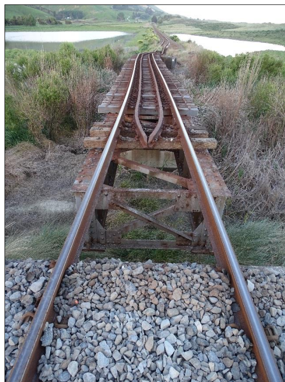
Major horizontal and vertical movement of land near bridge
