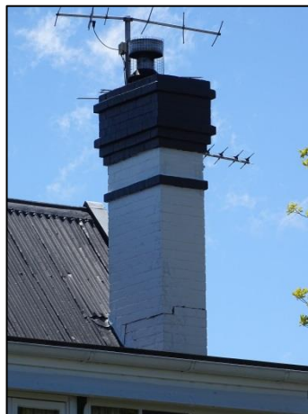
Horizontal crack at the base, Blenheim
