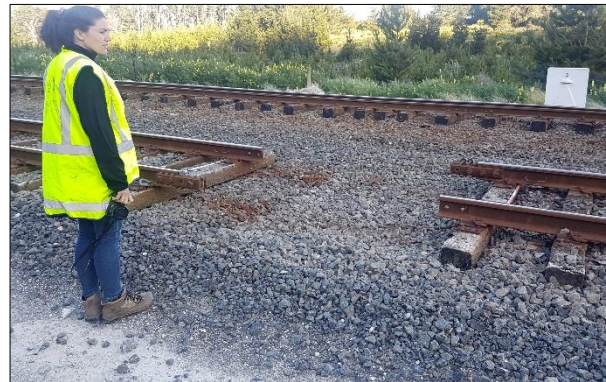
Shear failure and spread of railway lines
