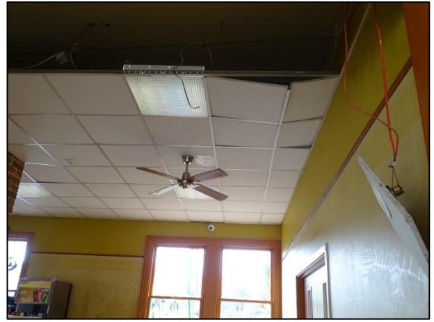
Ceiling damage due to chimney
