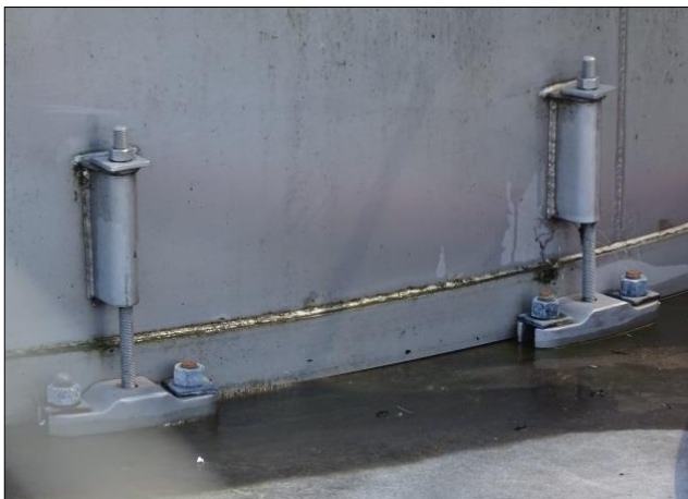
Evidence of movement and losing of connections
