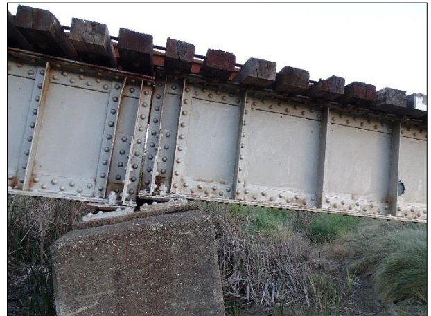
Close up of pier rotation
