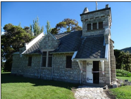
St Oswald's Church, stone and concrete, collapse of parts of front parapet
