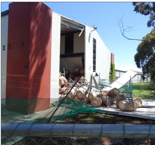
Collapse of stacking systems - wooded barrels' storage
