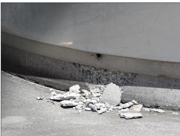
Shear failure of tank connections
