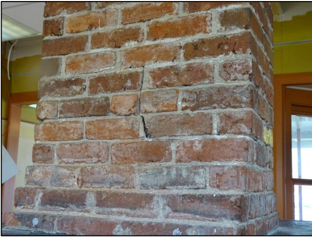
Chimney internal stack, torsional damage
