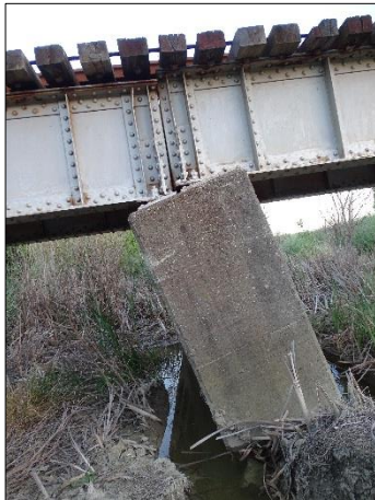
Major railway bridge pier rotation
