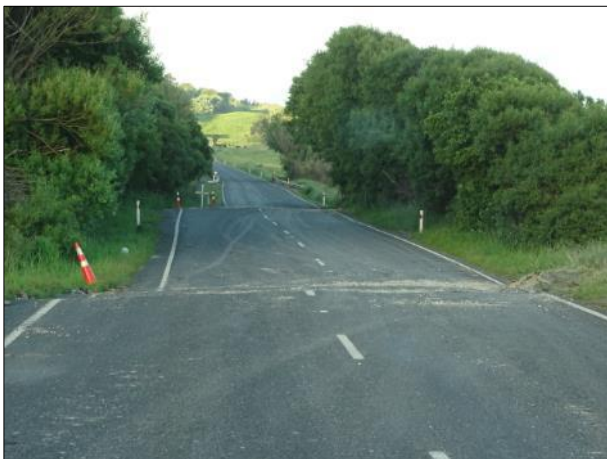
Significant vertical and horizontal shifts in road alignment
