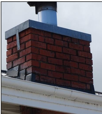
Dislodgement of the bricks, Blenheim
