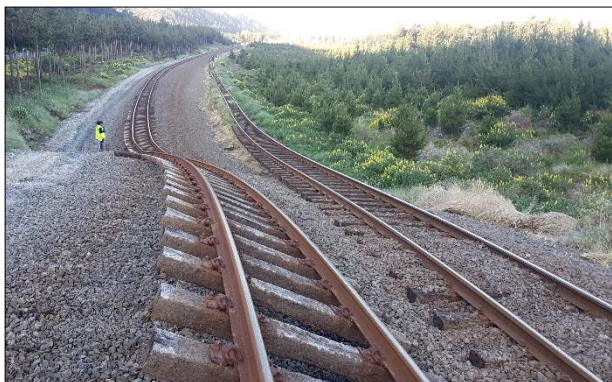
Major lateral displacement of railway lines
