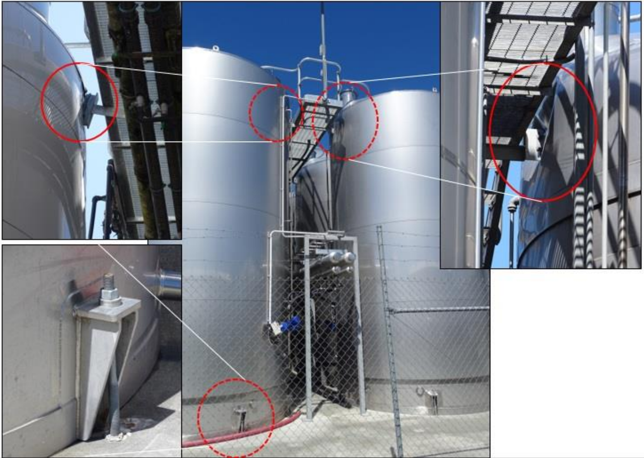
Damage to the walking platforms atop of tanks and anchoring connections due to tank movement
