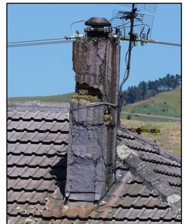
Extensive damage of the plaster, Blenheim
