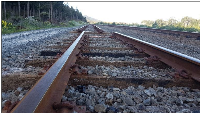
Rupture of railway lines at bolted joints – horizontal translation
