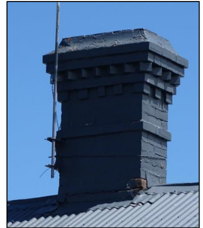
Horizontal crack at the roofline, Blenheim
