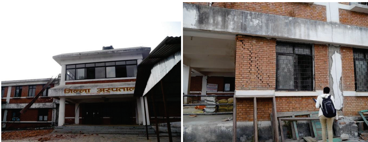
Figure 7 Main hospital building with heavy earthquake damage.
