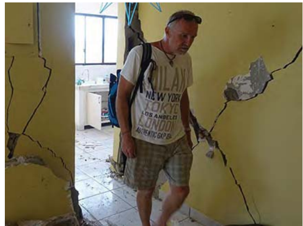
Figure 16. Damaged plaster and infills
