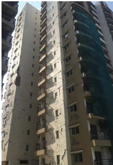
Figure 7. Exterior cracking, tower
