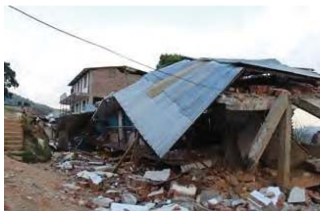
Figure 4. Collapsed school building
