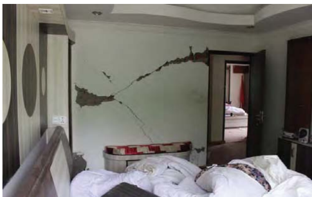
Figure 8. Interior diagonal cracking of infill walls
