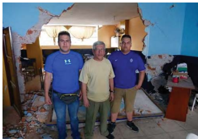
Figure 13. Infill wall failure school building
