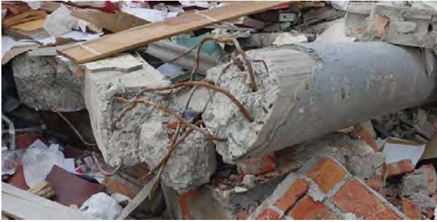
Figure 17. Poor detailing of reinforced concrete
