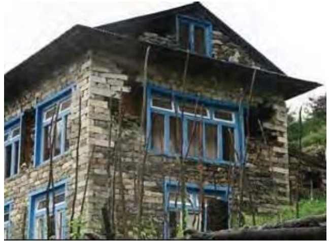
Figure 5. Out-of-plane failure of wall building
