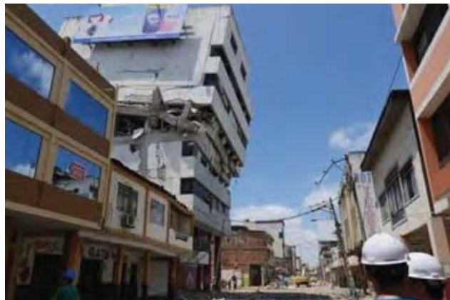
Figure 12. multi story damaged building
