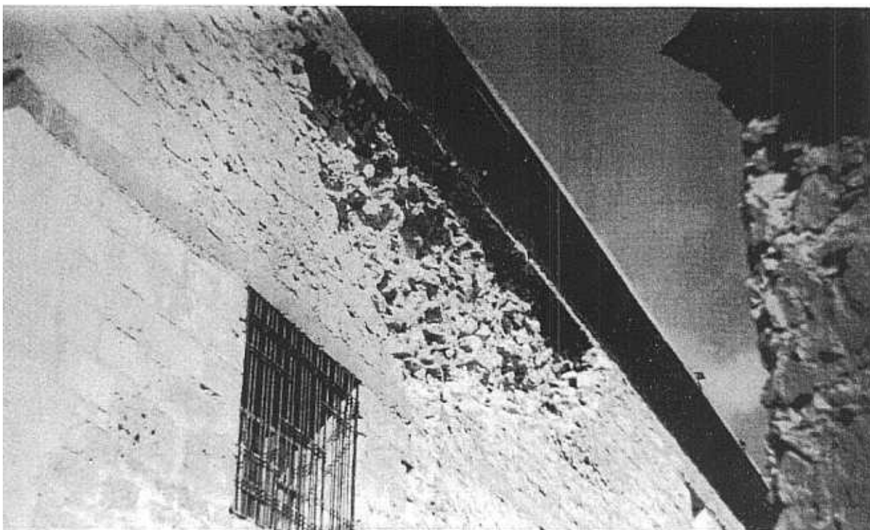
FIGURE THE START THE FAILURE WAL CEMENT MORTAR ICE
