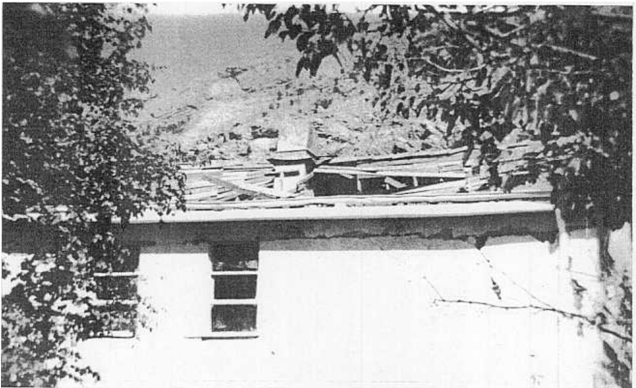
FIGURE 26 SEVERAL BRICK CHIMNEYS FELL THROUGH THE ROOFS OF THE HIGH SCHOOL BUILDINGS.
