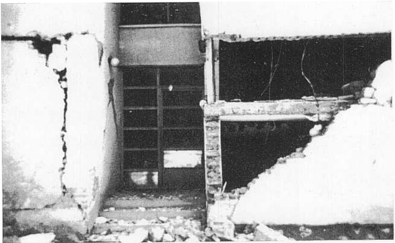
FIGURE 30 DAMAGE AND DEBRIS NEAR AN ENTRANCE TO THE HIGH SCHOOL BUILDING SHOWN IN FIGURES 28 AND 29.
