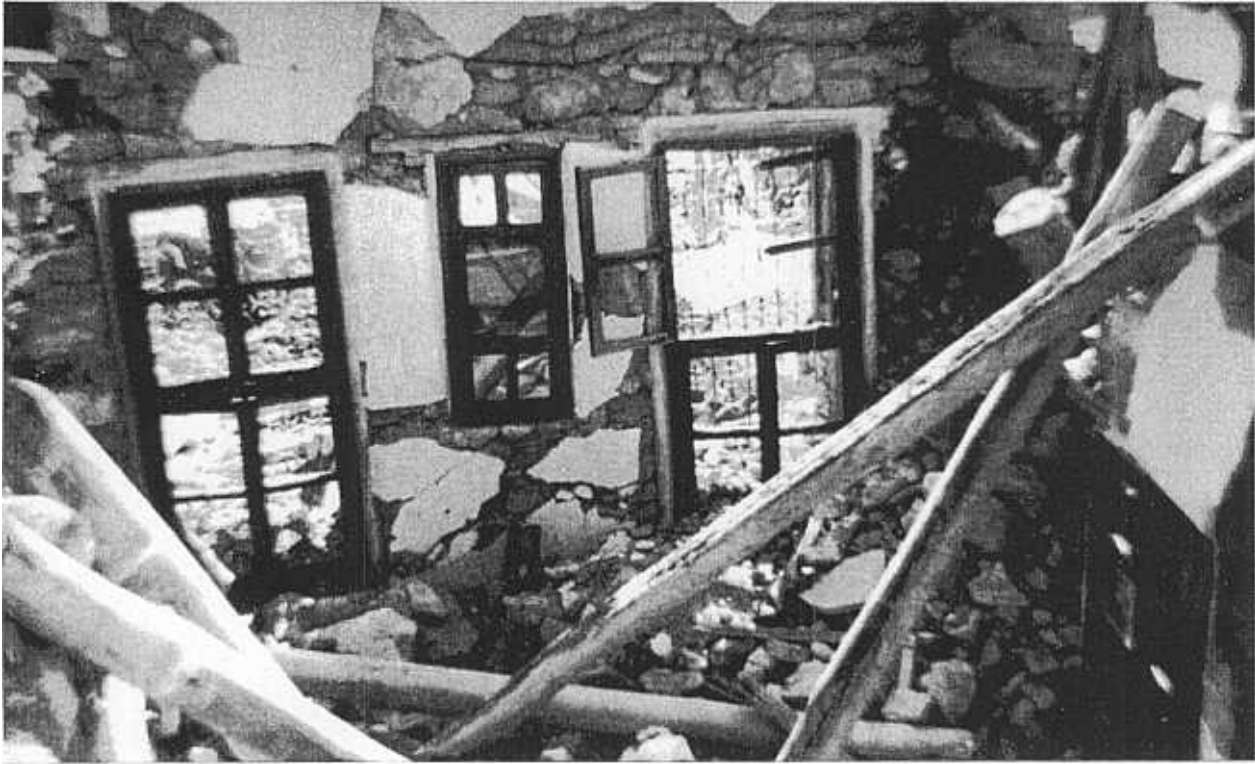
FIGURE INTERIOR A SEVEREL DAMAGED HOUSE LICE
