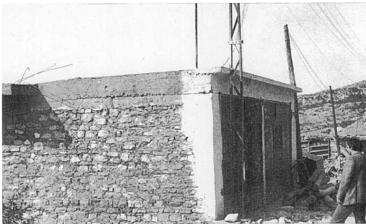
FIGURE 58 A LIGHTLY DAMAGED MASONRY COMMERCIAL STRUCTURE IN LICE, WITH A CONCRETE FLAT SLAB ROOF. SOME OF THESE BUILDINGS HAD CEMENT MORTAR.
