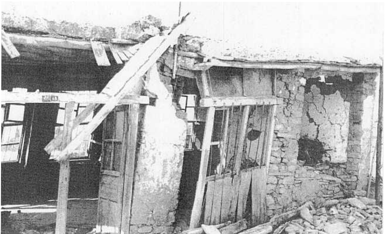
FIGURE 68 EXTERIOR OF A SEVERELY DAMAGED HOUSE IN LICE.
