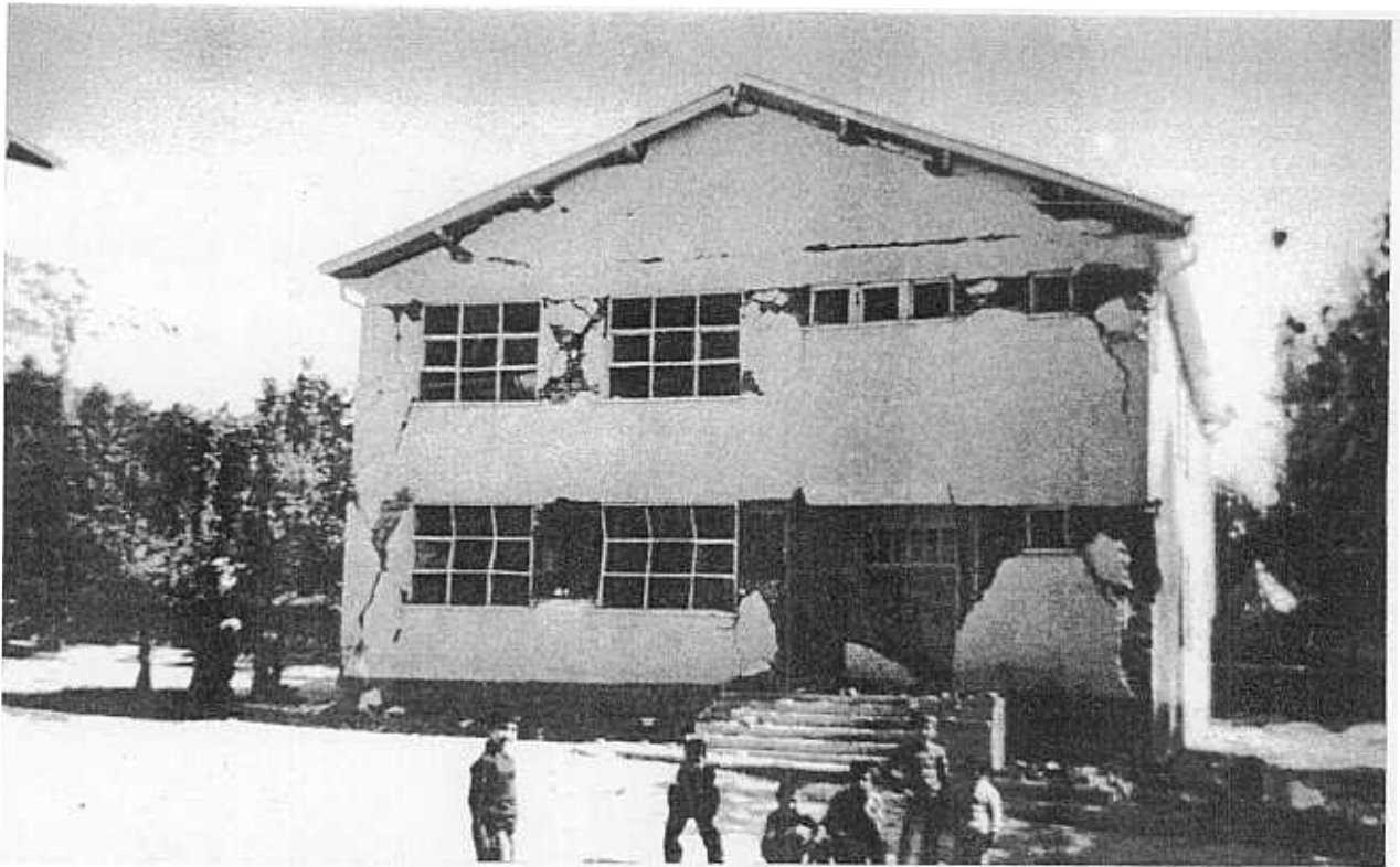
FIGURE 25 THE WEST WALL OF THE HIGH SCHOOL BUILDING SHOWN IN FIGURES 23 AND 24. AGAIN, ALL LATERAL RESISTING ELEMENTS ARE SHATTERED.
