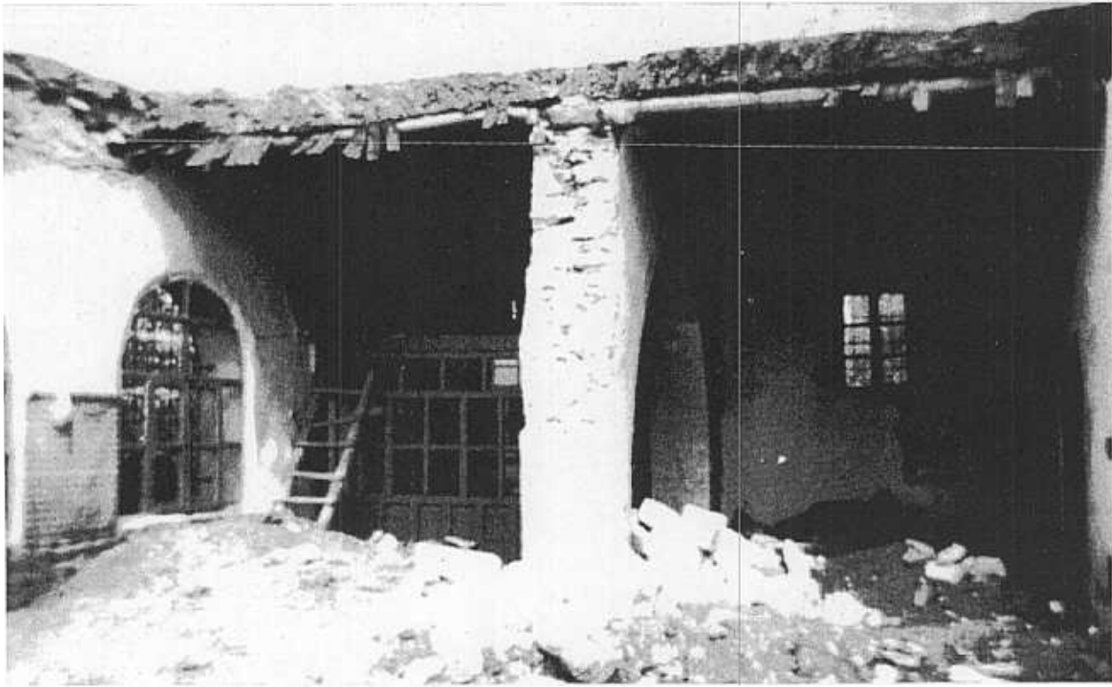
FIGURE 53 THE FAILURE OF INTERIOR LOAD-BEARING ARCHES IN THIS MOSQUE IN HANI LED TO THE COLLAPSE OF ITS HEAVY MUD ROOF.
