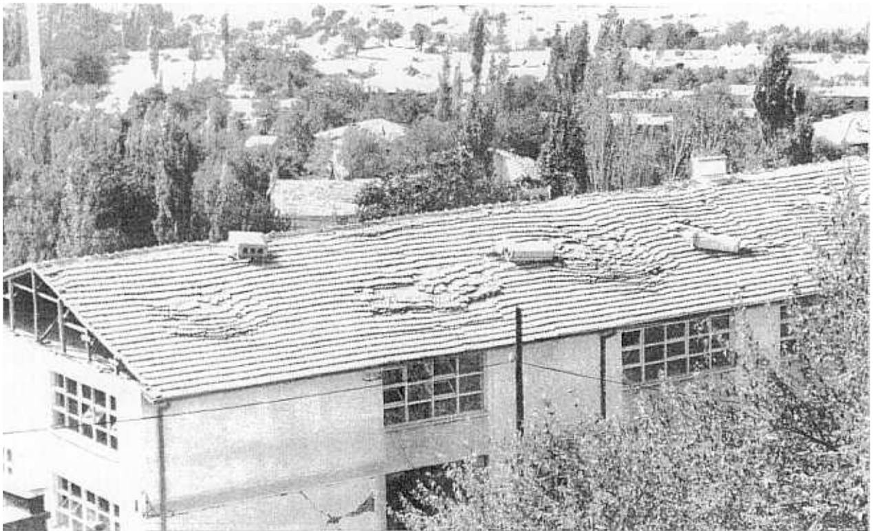
FIGURE 34 DAMAGE CAUSED TO THE ROOFING TILES, APPARENTLY BY AMPLIFIED VERTICAL VIBRATION IN THE CENTRAL AREAS OF THE HORIZONTAL ROOF SPANS BETWEEN THE VERTICAL TRUSSES.
