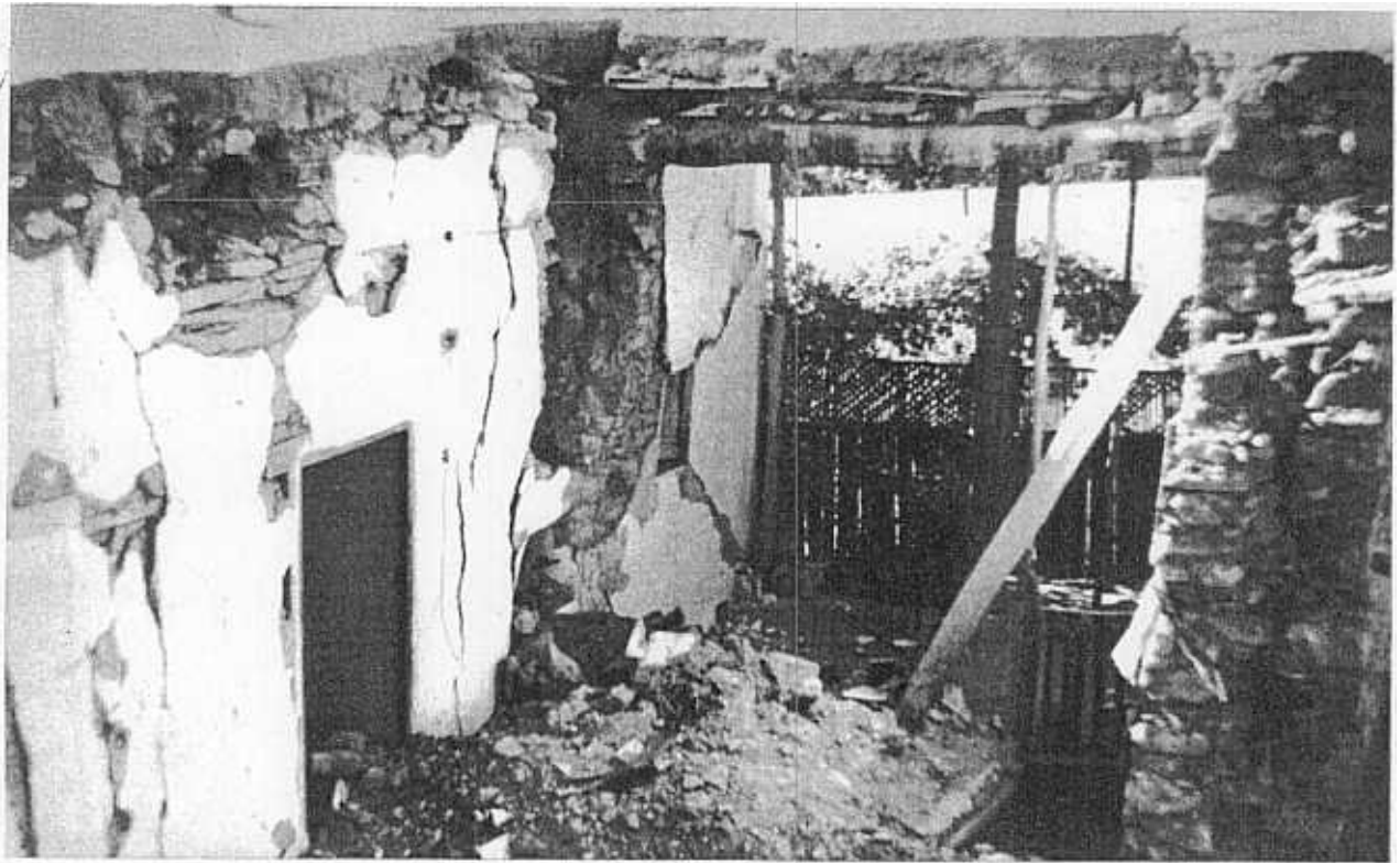
FIGURE 55 THE INTERIOR OF A HOUSE WITH A COLLAPSED ROOF IN LICE.
