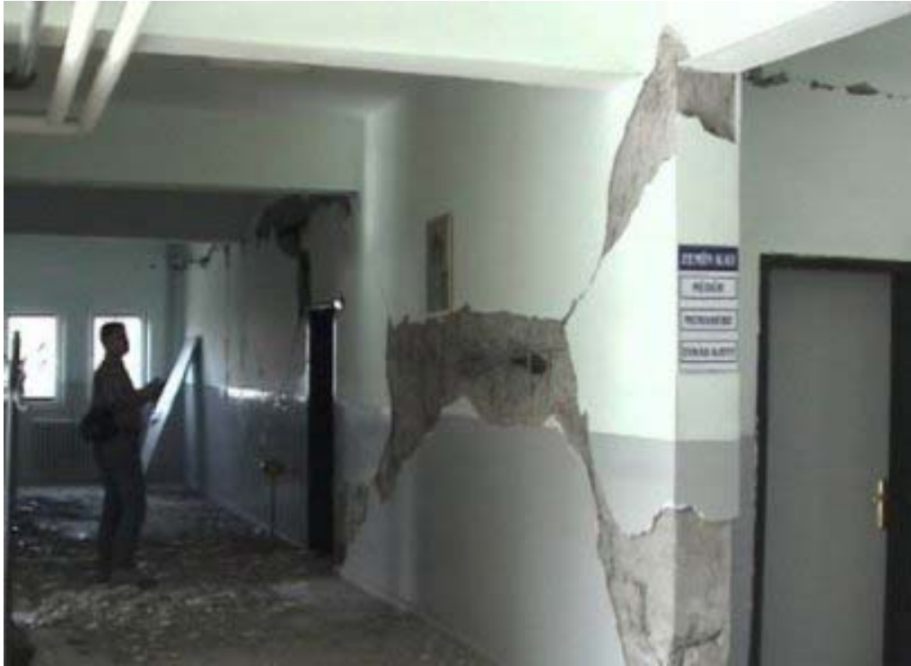
Figure 33. Observed shear failure at shear wall due to insufficient transverse reinforcement and poor concrete quality.
