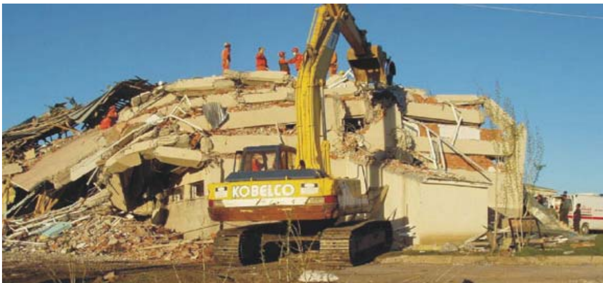
Figure 41. Pancaked Çeltiksuyu Primary School Dormitory (After Emre et.al, 2003)
