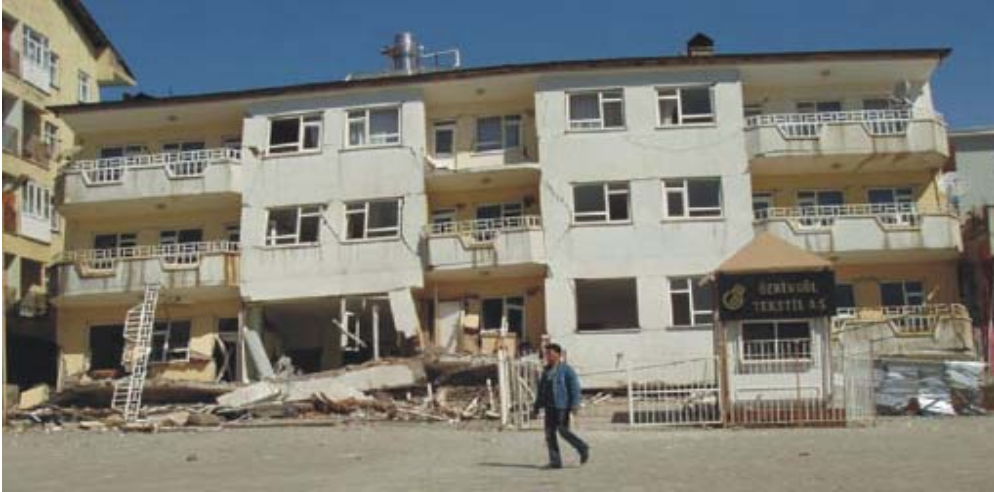
Figure 39. Typical First Story Collapses
