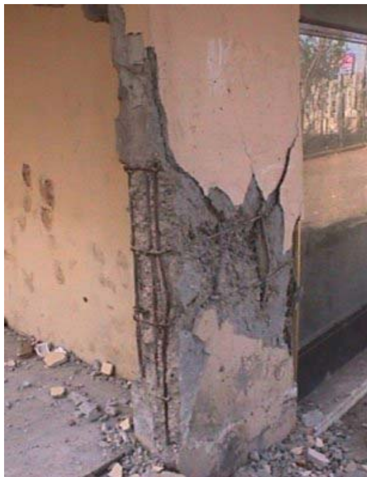
Figure 34. Shear failure at column base due to insufficient amount of transverse reinforcement
