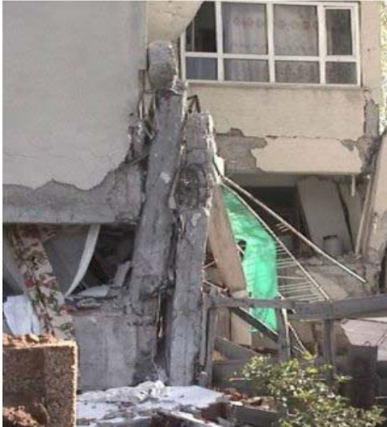
Figure 37. Collapsed first two stories
