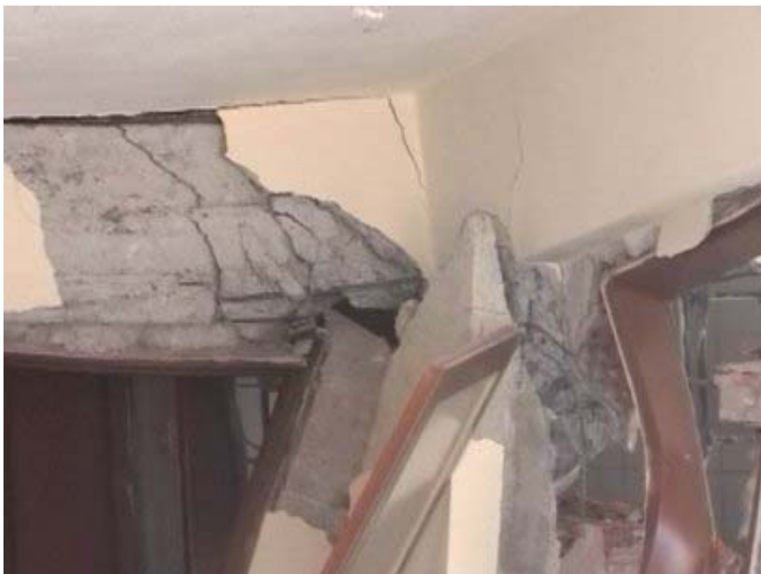
Figure 35. Typical shear crack at beam end
