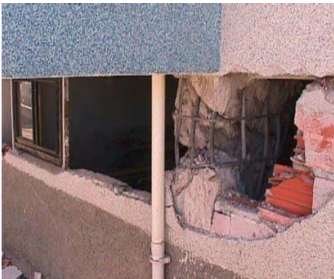
Figure 36. Shear failure at short column.
