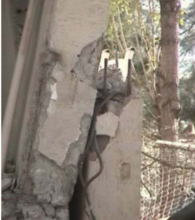
Figure 38. Insufficient development length at the top of column
