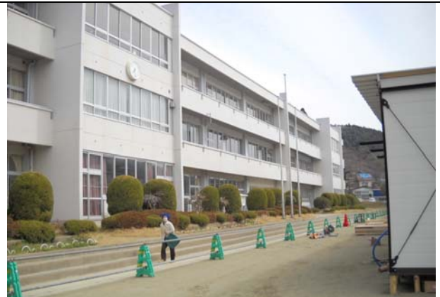
Photo 2: No damage in the school building.
