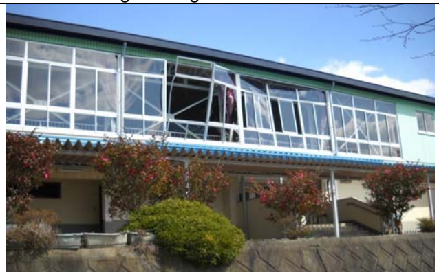
Photo 9: Window glasses were broken in the gymnasium (2).
