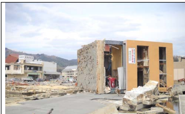
Photo 41: Overturned RC buildings (1).
