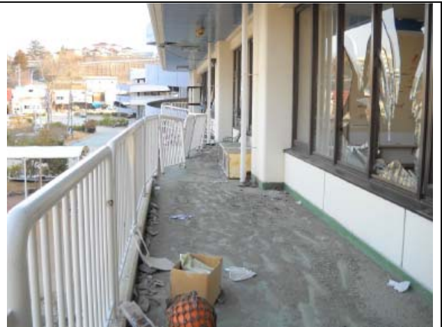
Photo 29: Window glasses and hand rail in the second story were broken.
