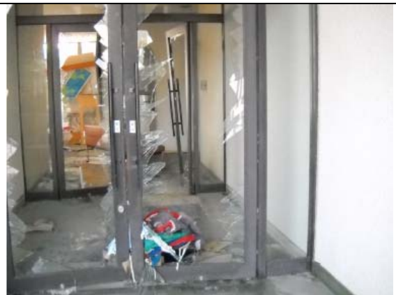
Photo 27: Glasses in the first story door were broken by tsunami wave.
