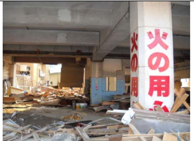
Photo 32: The first story of the fire station building (content was severely damaged).
