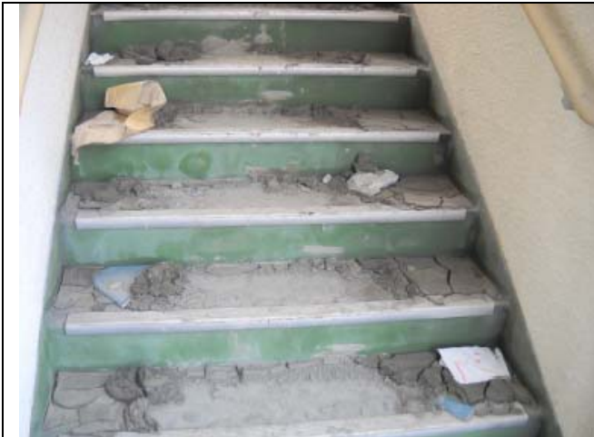
Photo 28: Stairs leading to the second floor were covered with soil.
