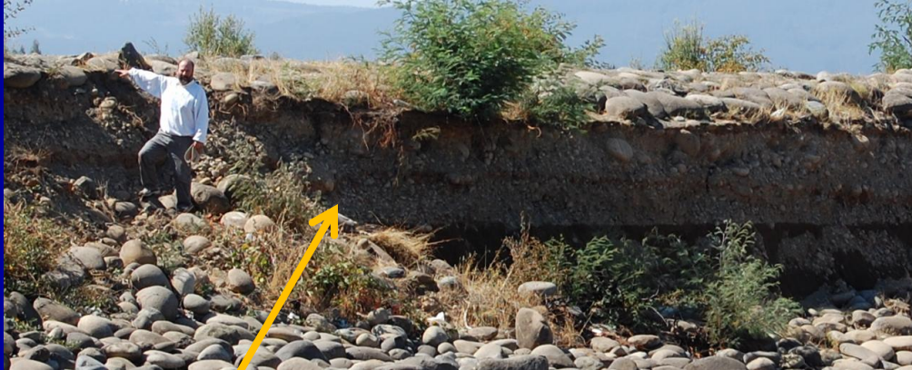
Coihueco Zoned Earth Dam Upstream Slope Failure
